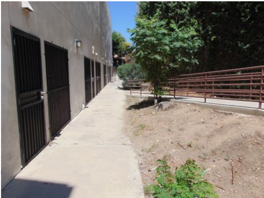
Photograph No. 6: View facing north along the exterior doors to the basement storerooms.
