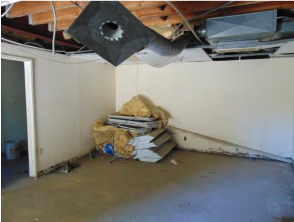
Photograph No. 9: A typical interior view of one of the basement areas.
