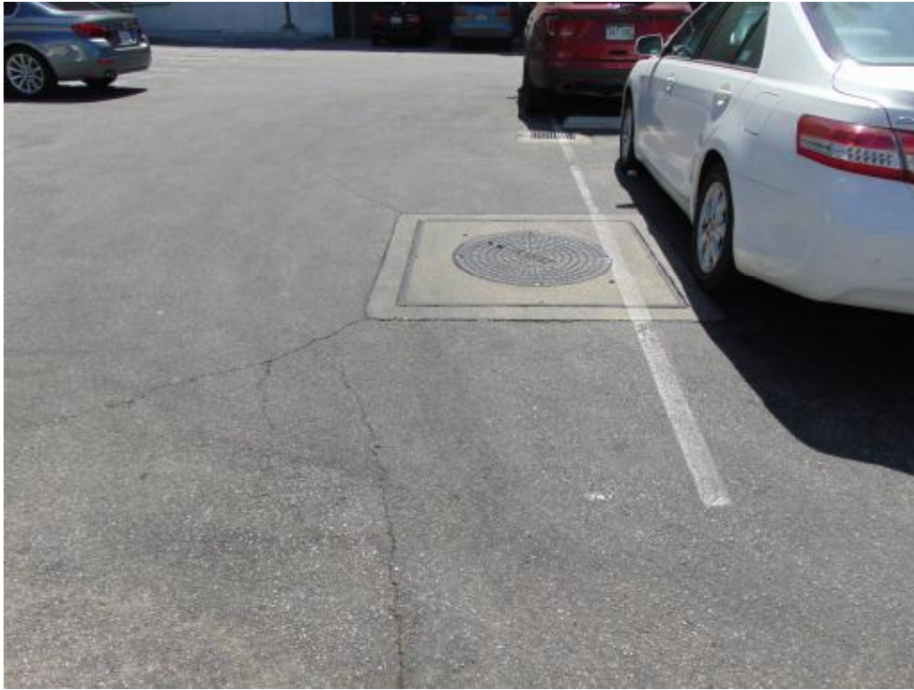
Photograph No. 11: An LADWP transformer vault in the front parking lot.
